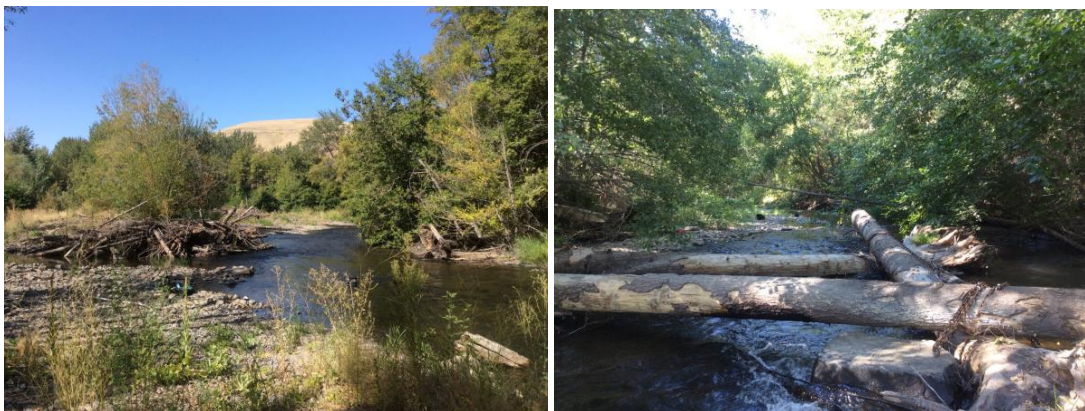
Figure 11. Photos showing two of 61 LWD structures constructed in Project Area 24. CHaMP post-treatment sample not available for this report.
