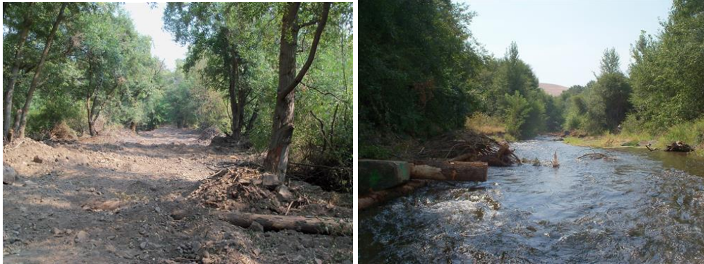
Figure 10. Restoration actions implemented in Project Area 23 included levee removal (left photo) and installation of LWD structures (right photo). Photos courtesy of the SRSRB. CHaMP post-treatment sample not available for this report.
