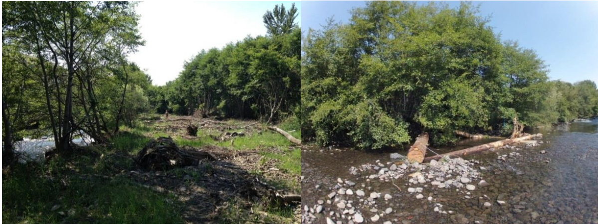
Figure 12. Restoration actions implemented in Project Area 26 included levee removal (left photo) in 2011 and LWD placement (right photo) in 2012. Photos courtesy of the SRSRB.
